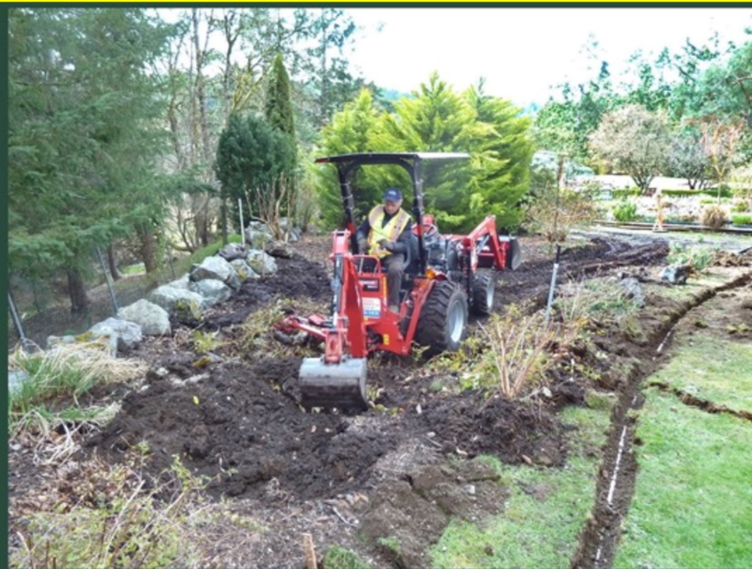
Day 1 - removal of plants, boulders and soil to a depth of 38", preparatory for 3/4" road base substrate for pavers and walls
